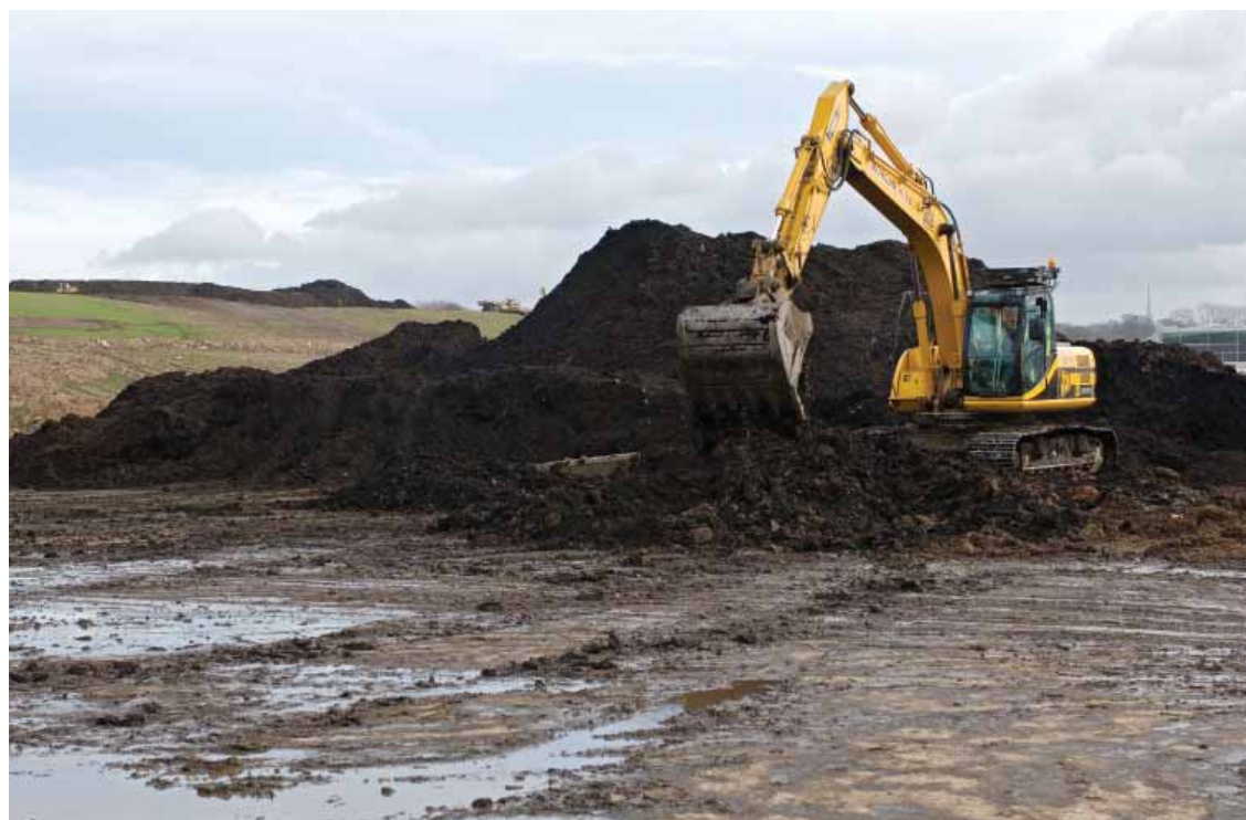
Land remediation in action at the British Aerospace former Royal Ordnance facility in Chorley
